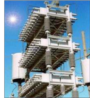
Open Rack Shunt Banks
