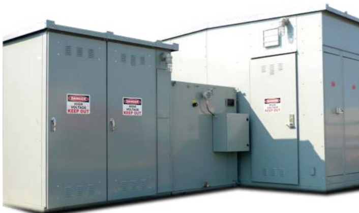
Metal Enclosed Capacitor Bank Equipment
