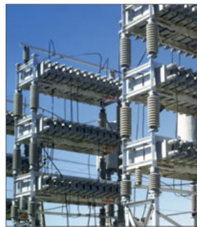
Open Rack Harmonic Filter Bank
