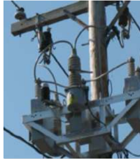
Pole Top Shunt Banks
