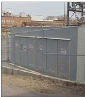
Metal Enclosed Shunt or Filter Bank
